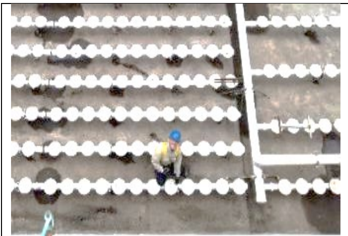
Photo: Existing air diffuser system
