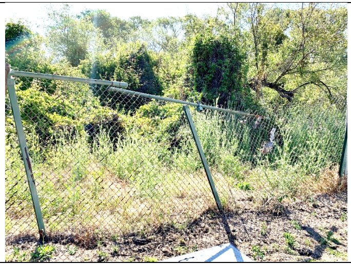
Photo: Existing Dilapidated Fence
