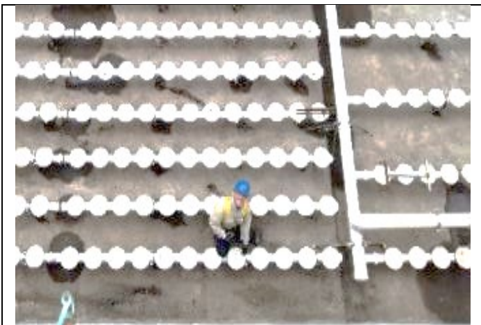
Photo: Existing air diffuser system
