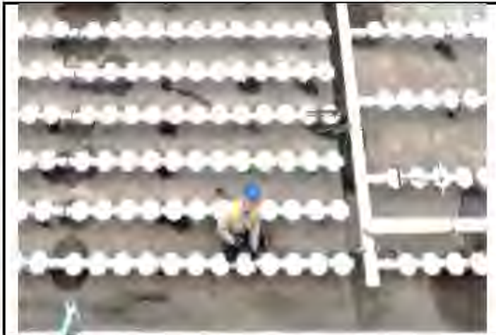
Photo: Existing air diffuser system
